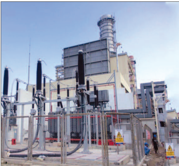
Ghorashal Power Plant
